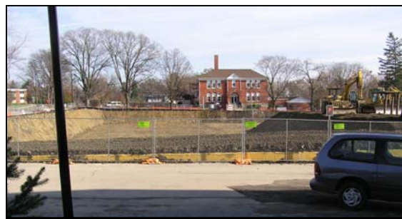
The foundation dug for the new science building. Looking from the Beamer Center and Coray Gym toward Jenks.
